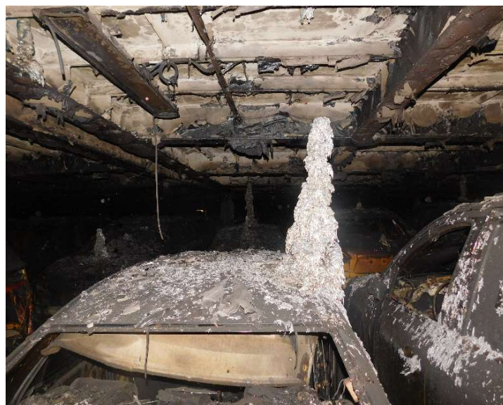
Figure 4. Deck 7 of the HOEGH XIAMEN taken on June 26, 2020, provided by the Coast Guard.
